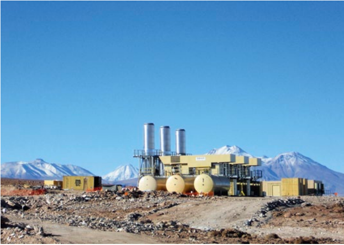
The multi-fuel power generation system comprises three turbines each with a capacity of 3.8 MW.
