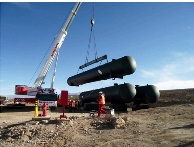
The liquefied petroleum gas storage facility for the generation system consists of three 200 m 3 tanks.
