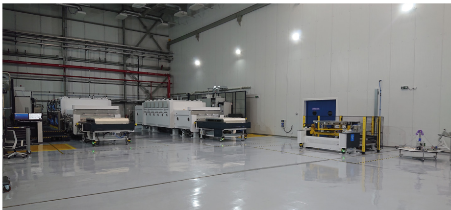
The installation of the first M1 segment coating plant started in February 2022 in the ETF at Paranal after more than a year and a half in storage because of the pandemic. By the end of the year, the two plants were operational. They will be used to coat the M1
