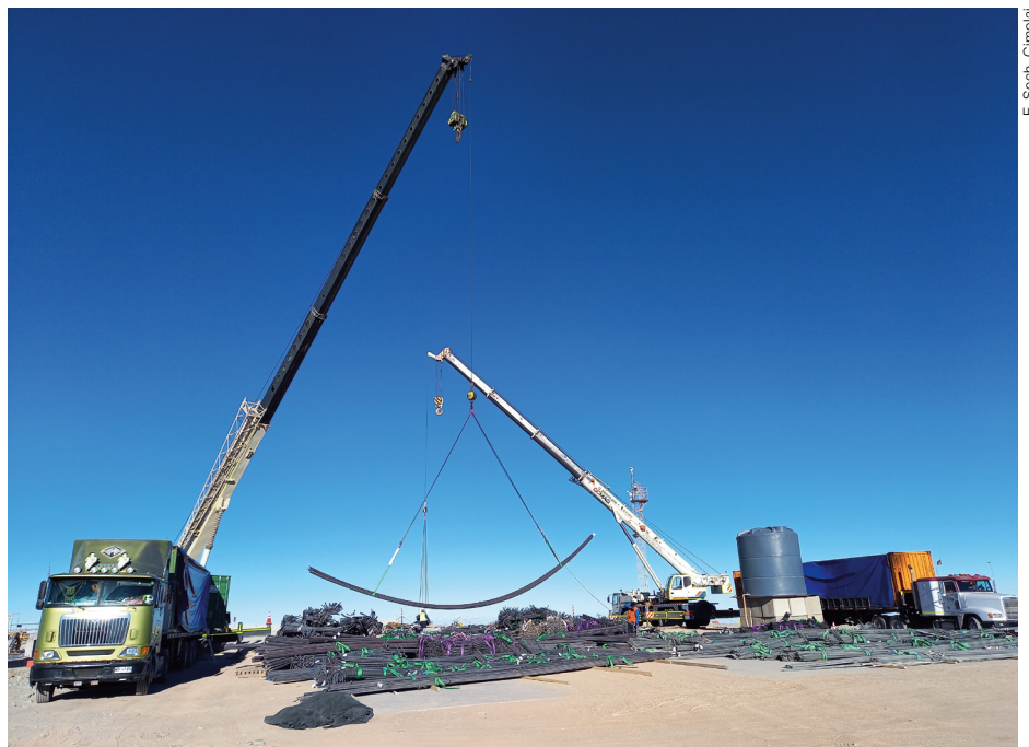
Handling of material and equipment received from Europe for the ELT Dome and Main Structure, Cerro Armazones.
