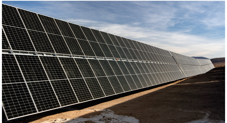
A row of solar panels at the Paranal–Armazones photovoltaic plant. This solar power plant has the highest generation capacity in Chile dedicated to astronomy.
