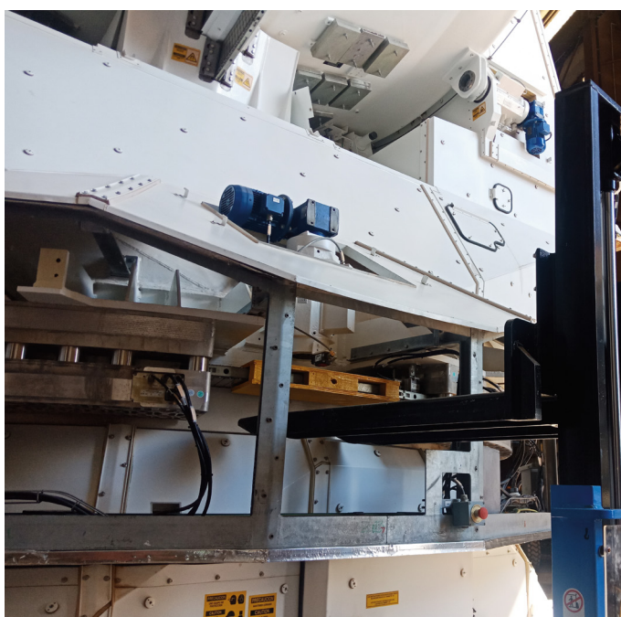
Removal of an azimuth motor segment that was found to be damaged during overhaul inspections of the ESO-provided ALMA antennas.
