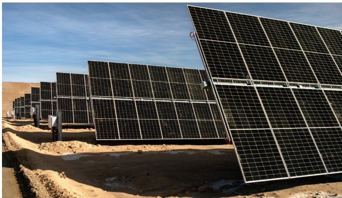
Rows of solar panels at the Paranal-Armazones photovoltaic plant.
