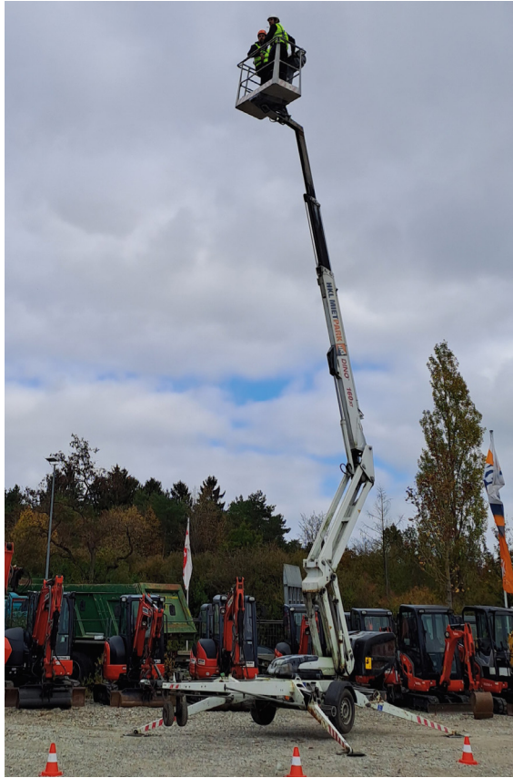
Training in the use of personal protective equipment for fall protection (left); operator training for a mobile elevating work platform (right).
