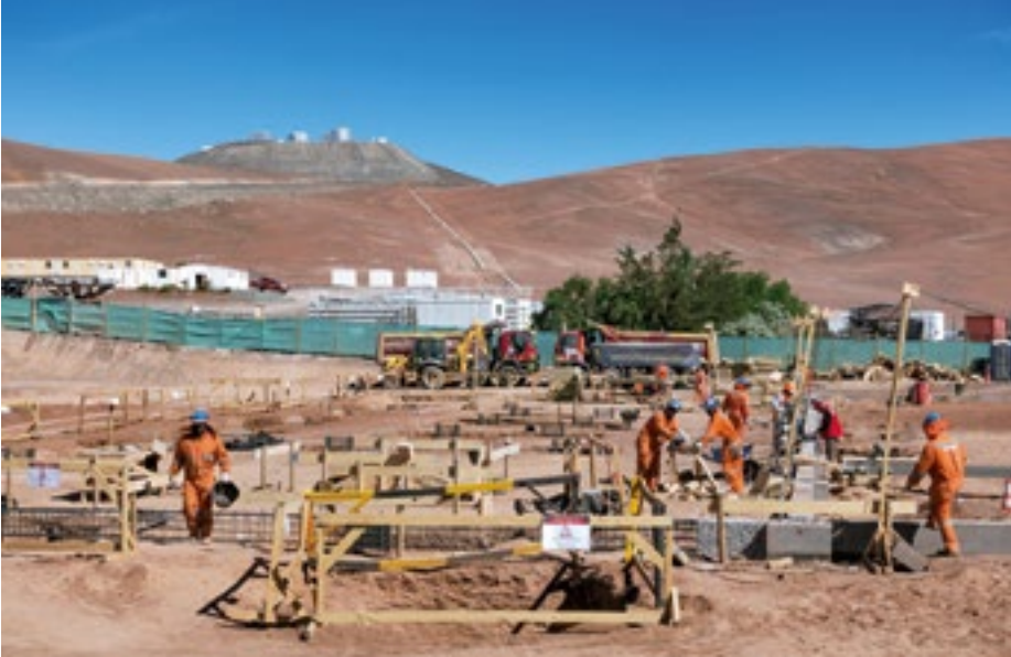
The future site of the Technical Facility for ESO's Extremely Large Telescope (ELT). The VLT can be seen in the distance.
