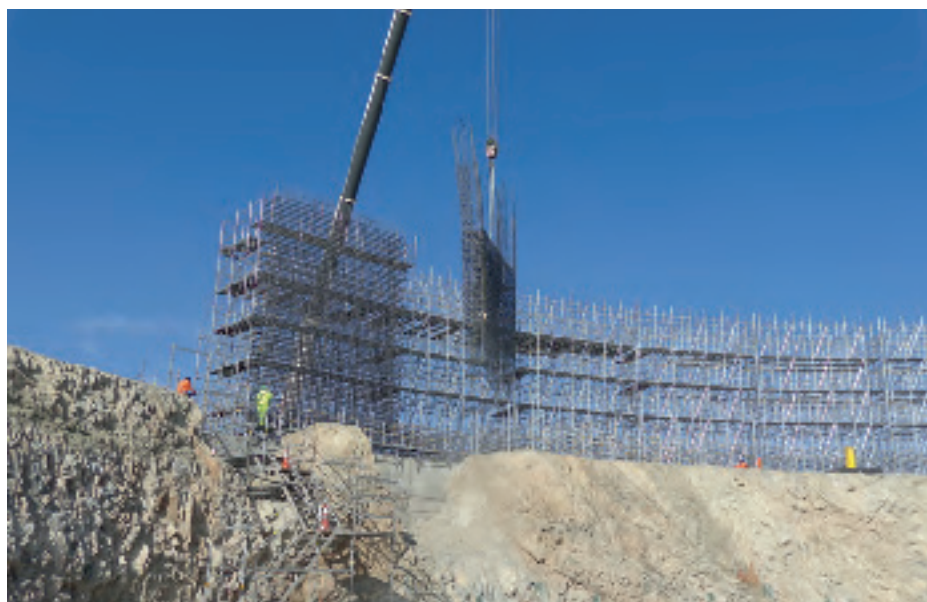
The ELT construction site at Armazones was closed in June 2020 because of the COVID-19 pandemic situation in Chile and re-opened in May 2021. By the end
