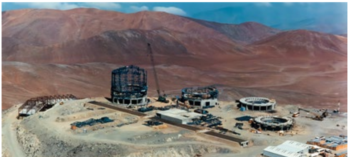
Top: The construction site of the VLT in 1996. Bottom: The VLT as it looks now.
