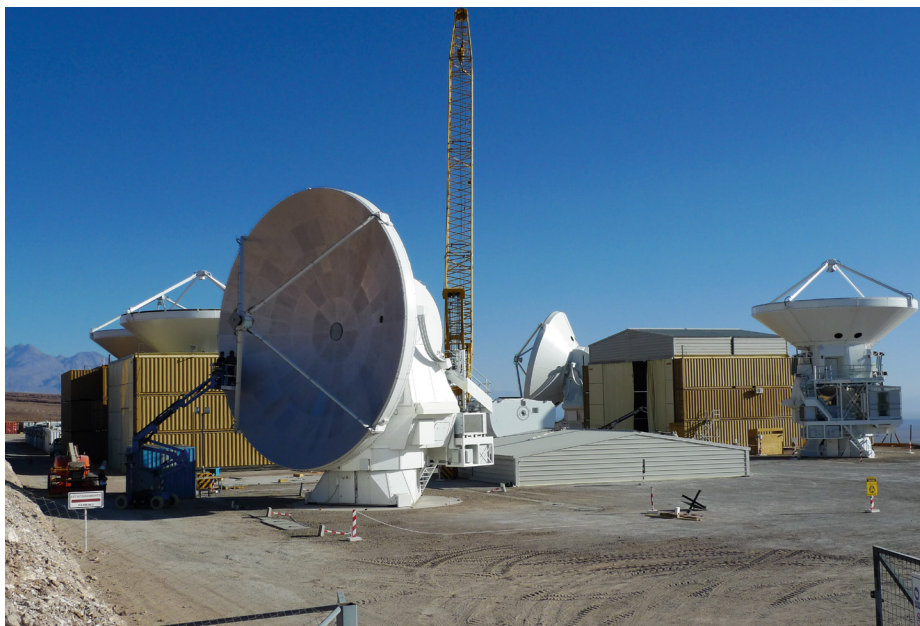
Figure 3. The AEM antenna camp at the OSF. Five antennas are fully assembled while a sixth is inside the temporary shelter on the right ready for the installation of the main reflector assembly; parts of the seventh antenna are also being assembled.
