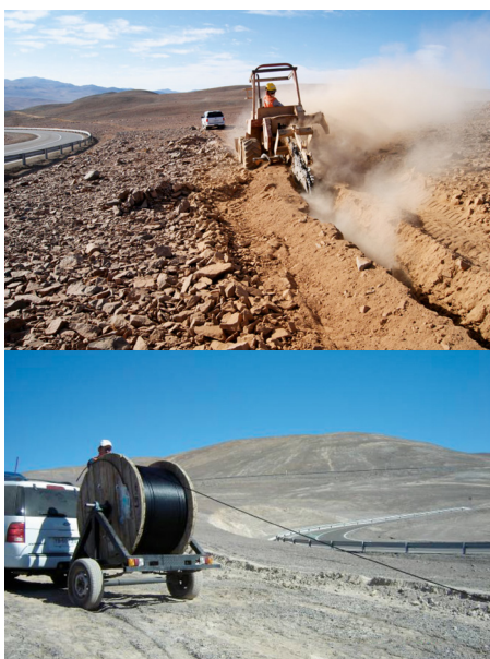
Figure 2. Two views of the work involved in laying the EVALSO optical cable from Paranal to link with the existing network infrastructure; upper image: cutting the trench; lower: laying the cable in the trench.
