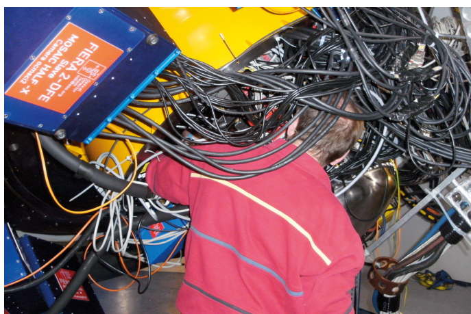
Figure 4. Cables, cables, cables... OmegaCAM behind the VST.
