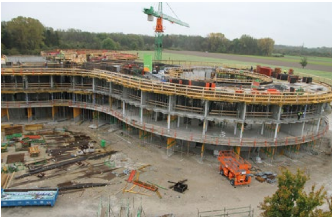
Construction of the extension to ESO Headquarters was begun at the beginning of this year and has now reached the second floor, as shown in this recent image. More details of the building concept can be found in a Messenger article (135, p. 2) and in Release eso1215.
