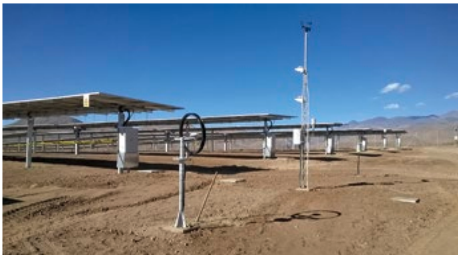
Figure 9. The new solar photovoltaic plant at La Silla.
