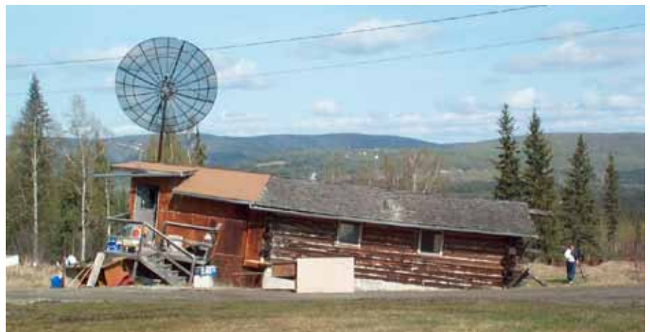
Figure 5: Infrastructure collapse due to thawing ice-rich permafrost terrain, Alaska, USA
